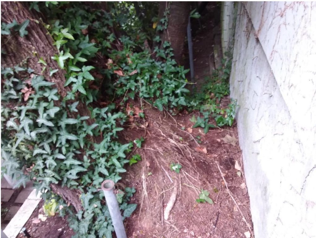
Figure 9. Showing the proximity of the subject garage to the base of the #3 tree.
