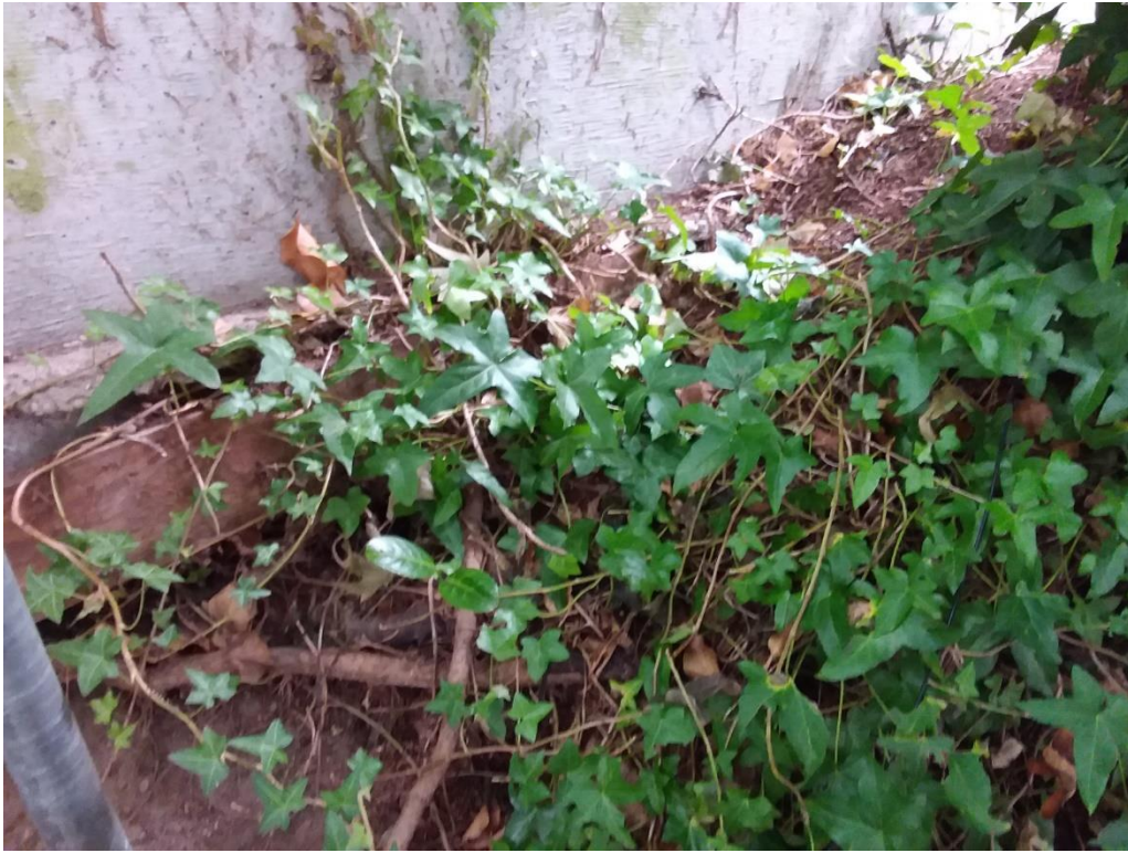
Figure 12. Looking at the base of the north side foundation/retaining wall of the existing garage. There is evidence that the #3 tree has roots growing under this section.
